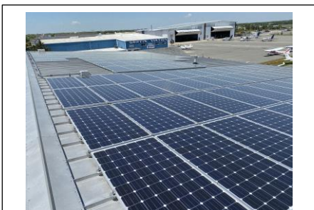
Rooftop Solar Array – Cape Air Rented Facility Cape Cod Gateway Airport
